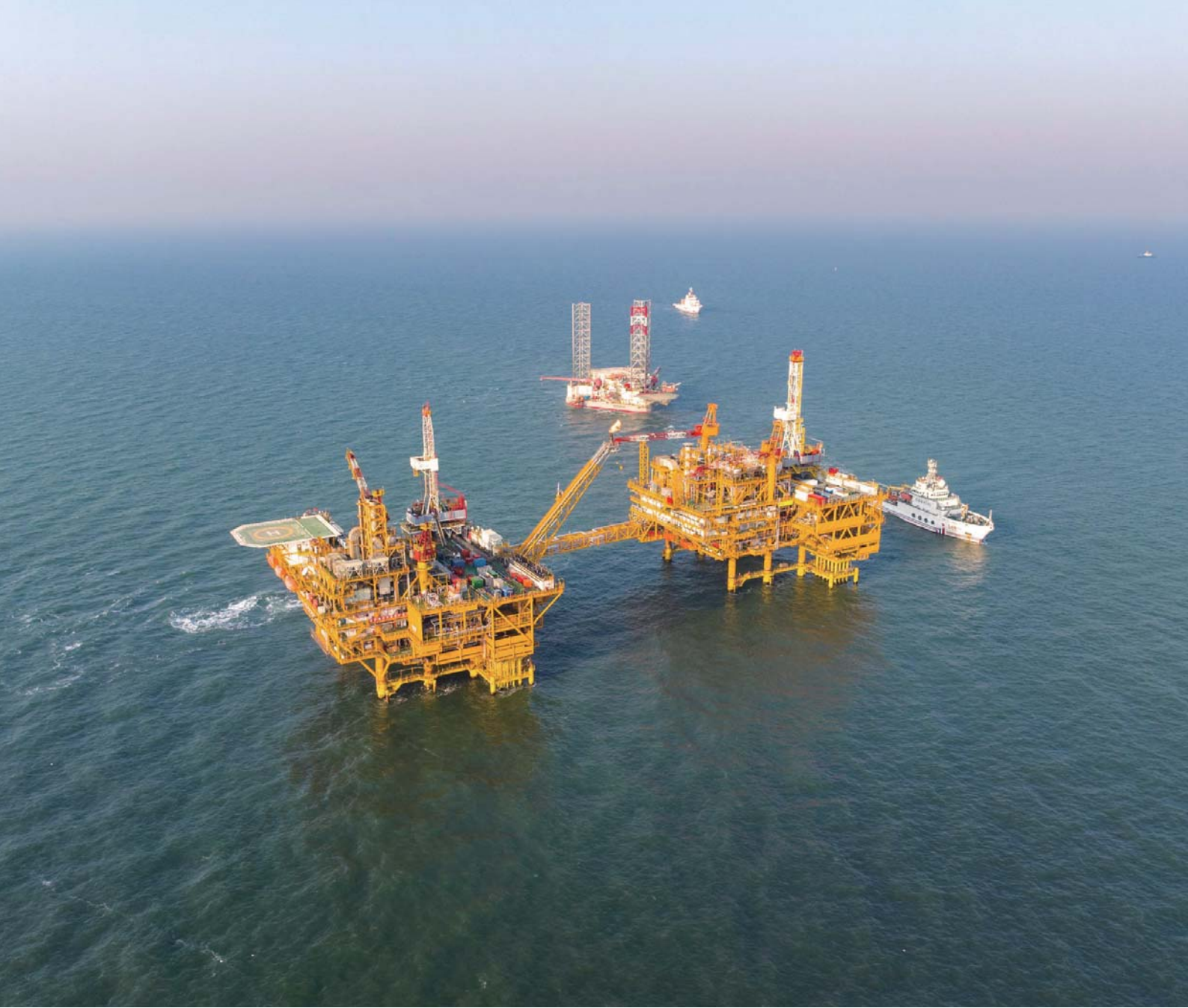
▲ Offshore installation of CEPB module is completed for Caofeidian 6-4 Oilfield Well Area Development Project
