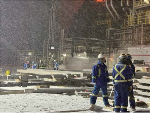
^ Several projects at the Canadian subsidiary, including Overhead Corrosion and Chemical Tank T17T58, are still in operation, with approximately 75 people working on-site. (Photo: Frontline workers assemble the main structural supports in heavy snow at -30°C on the Overhead Corrosion project site)
