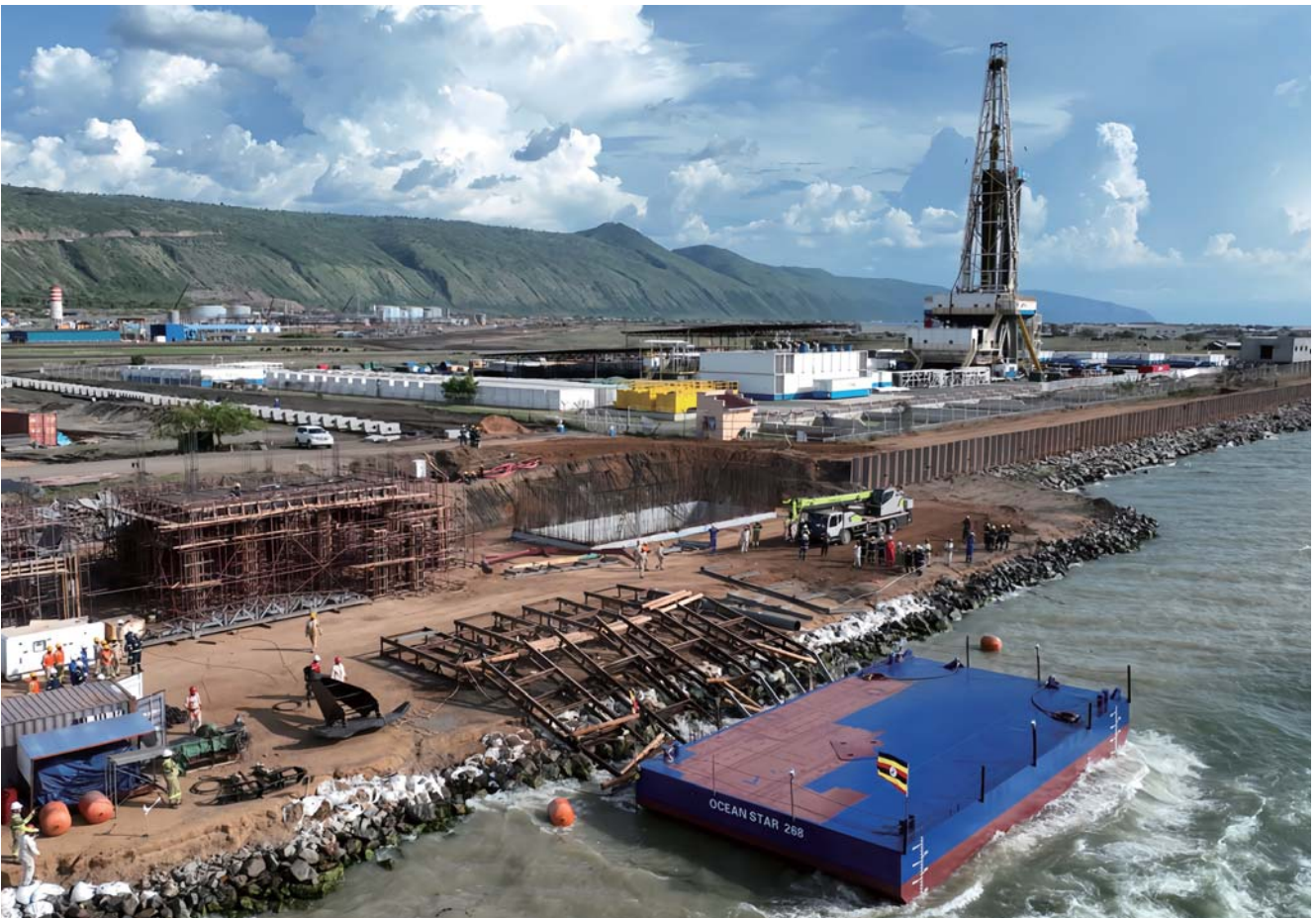
v The barge for the Kingfisher project in Uganda is successfully launched
